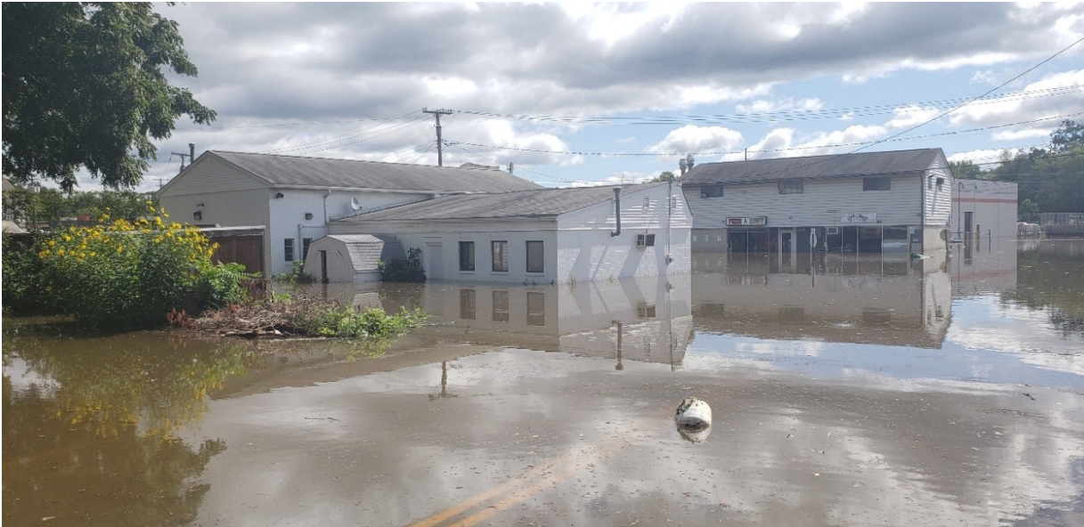
Flood damage in the Town of Fishkill, New York.
